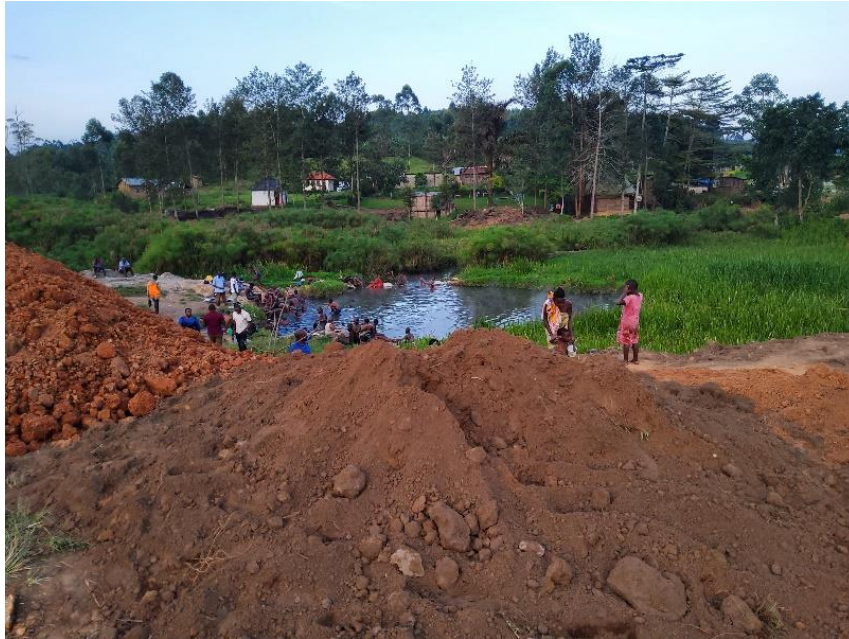
Figure 11: Civil works on-going at Kitagata (Ekyomugabe hot spring) as part of the geothermal spa development plan.
