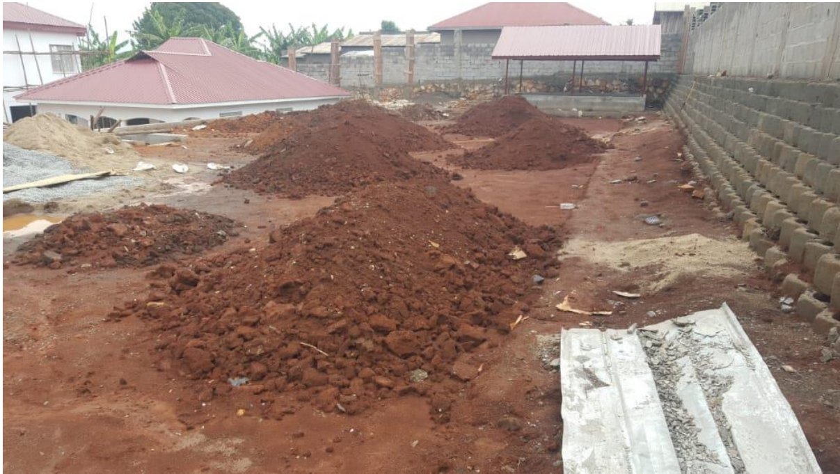
Figure 8: Progress on Fort Portal Beneficiation Centre construction. Structures and Perimeter wall already done, Leveling of compound was ongoing as of 30/06/2021.
