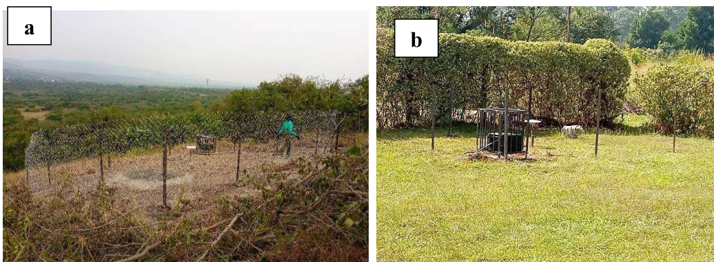
Figure 2: (a) GNSS observation station installed at Queen's Pavilion, QECA, Kasese (b) GNSS Observation Site installed at Hoima Seismic Station, Katasiha Site.
