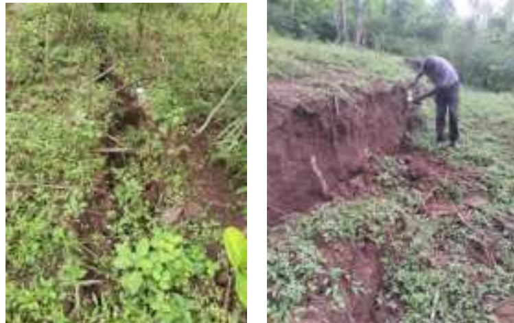
Figure 25: Crack and subsidence at Shibanga Village, Manafwa District.
