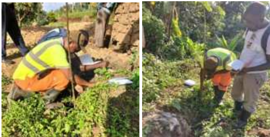
Figure 22: Geo-hazard assessment and geotechnical investigations of cracks in Nakitwe village, Kibanda Parish in Bulambuli District.
