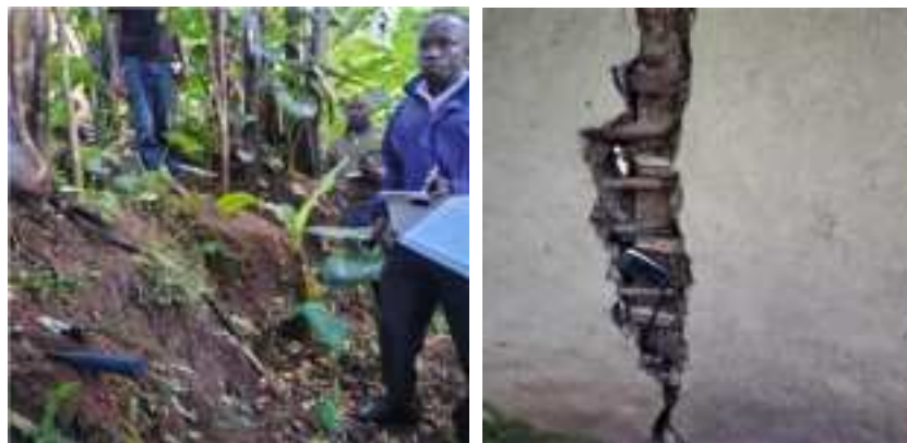
Figure 24: Subsidence causing house wall crack in Nachere Village, Bumboi Parish in Bududa District.
