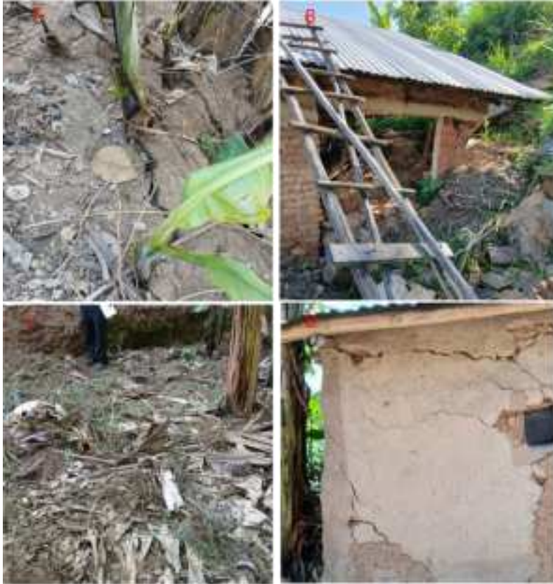
Figure 14: Shows indicators of slope failure with A showing developed cracks in the ground, B showing a house destroyed by the landslide, C showing ground subsidence & D showing a house with cracks running through it.
